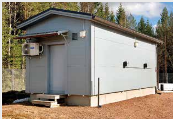
Steel-framed fire class P2 equipment shelter.
